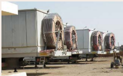
Al-Qaim mobile substations
