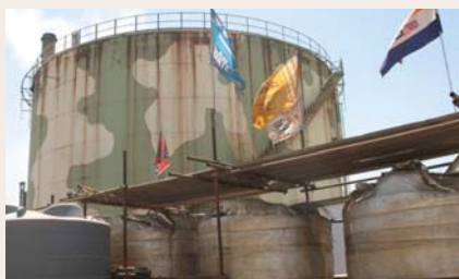
Doura power plant
