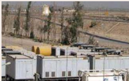
Generators at Baghdad International Airport
