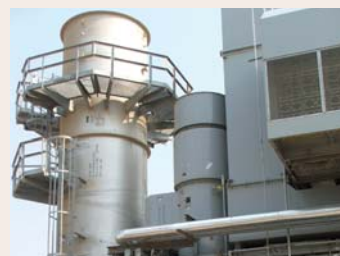
Qudas power plant
